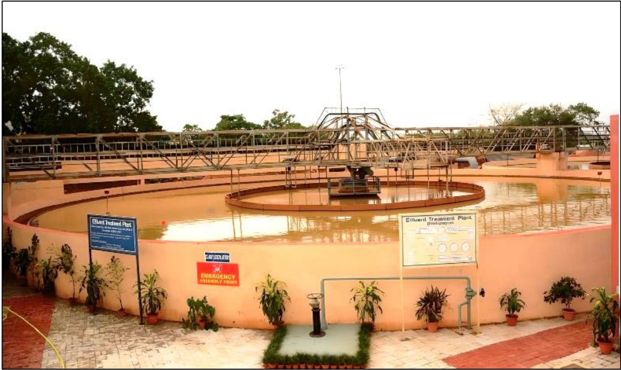
Chromite Mine Effluent Treatment Plant
