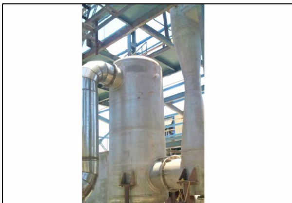
Secondary Combustion Chamber
