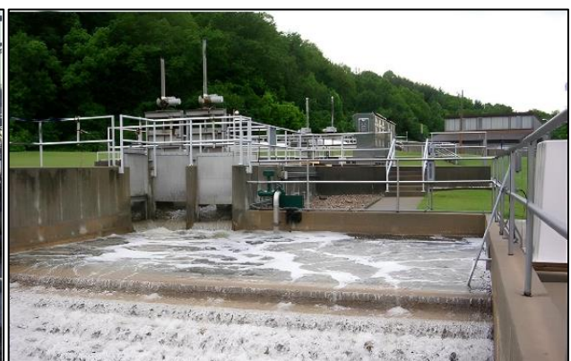
Sewage Collection Tank & Cascade Aerator
