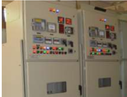
Indoor MV Switchgears upto 33 kV
