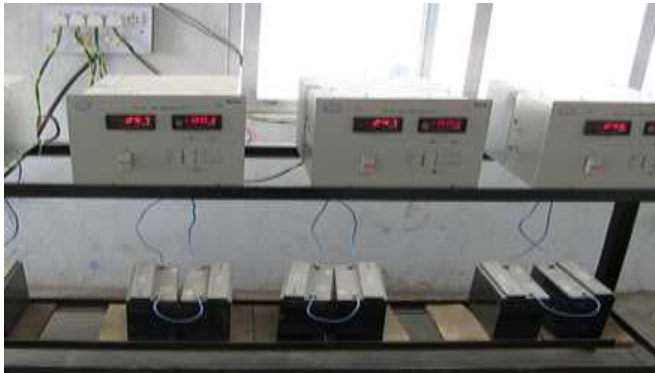
Battery and Battery Chargers
