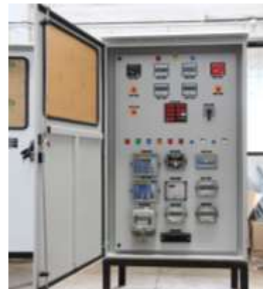
Control and Relay Panels
