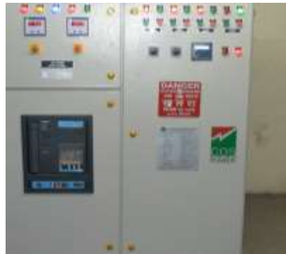
LT APFC (Automatic Power Factor Control) panels with contactor based switching
